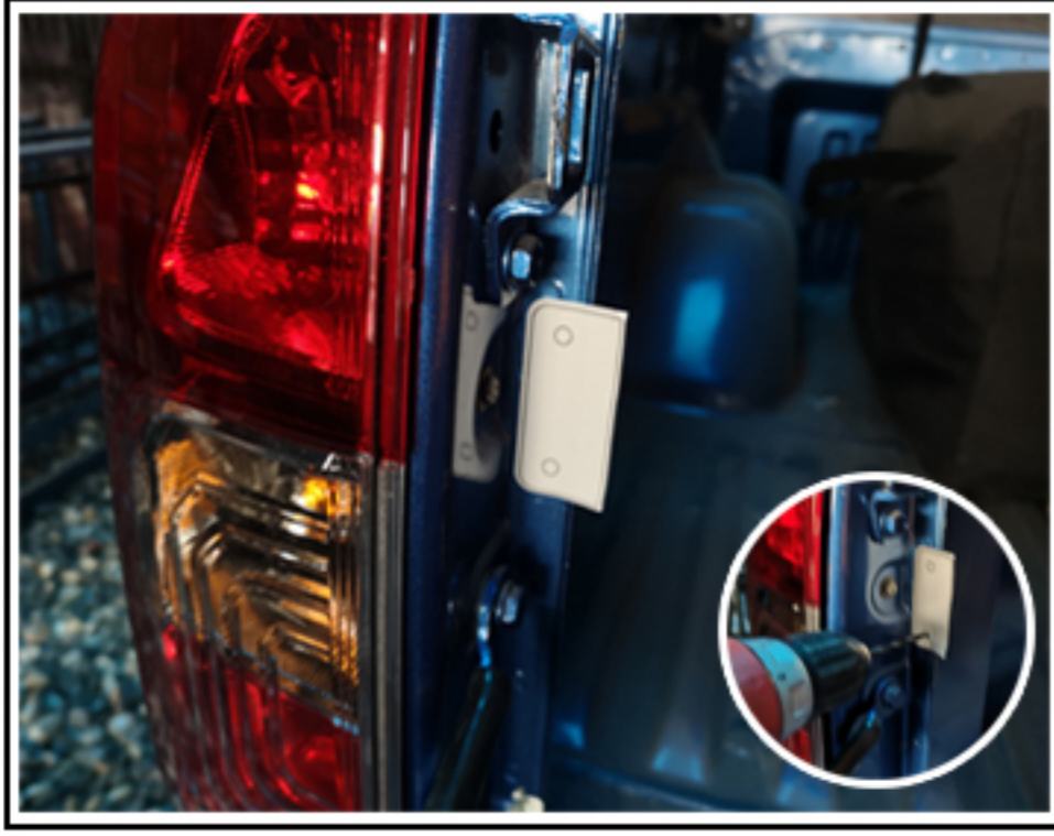
11. Stick the fixed position on the place where the expansion rack is installed, and punch holes according to the hole positions.
